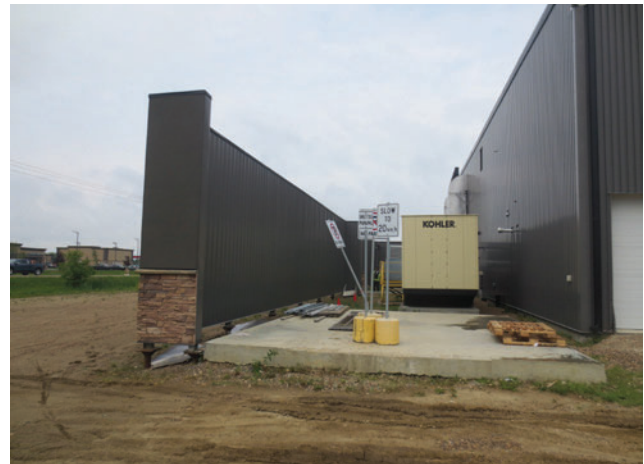
Equipment located back of house and screened near loading bays.
