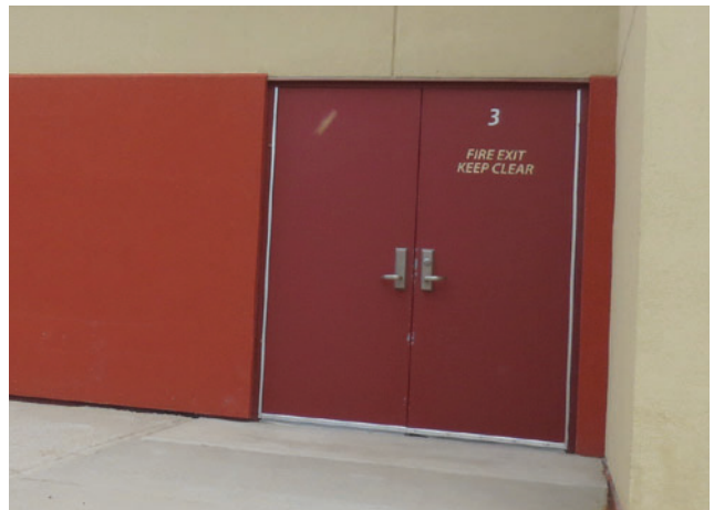
Doors numbered and labeled with Fire and Life Safety Purpose.
